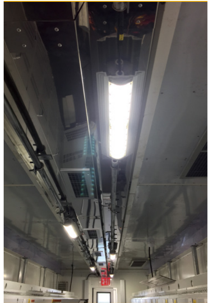
HDL2s in an electrical control room
