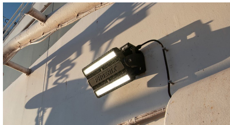
Deck and Crane Lighting
