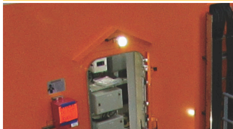
Emergency Battery Backup Lighting
