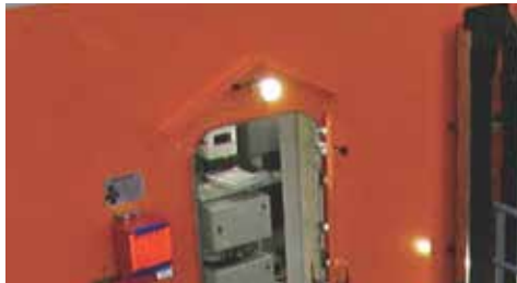
Emergency Battery Backup Lighting
