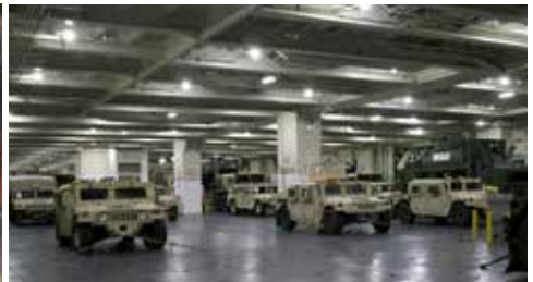
Cargo Hold Lighting
