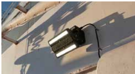
Deck and Crane Lighting
