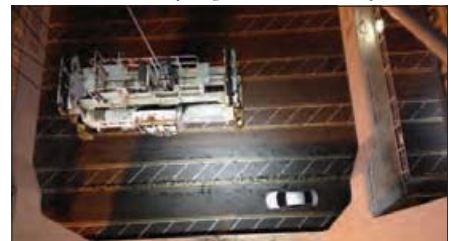
Phoenix ModCom Hi LED floodlights on an STS crane trolley
