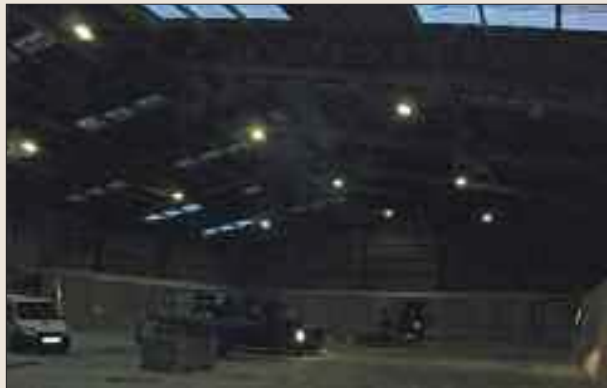
BEFORE: prior to a lighting overhaul the illumination of this Forth Ports' shed was weak
