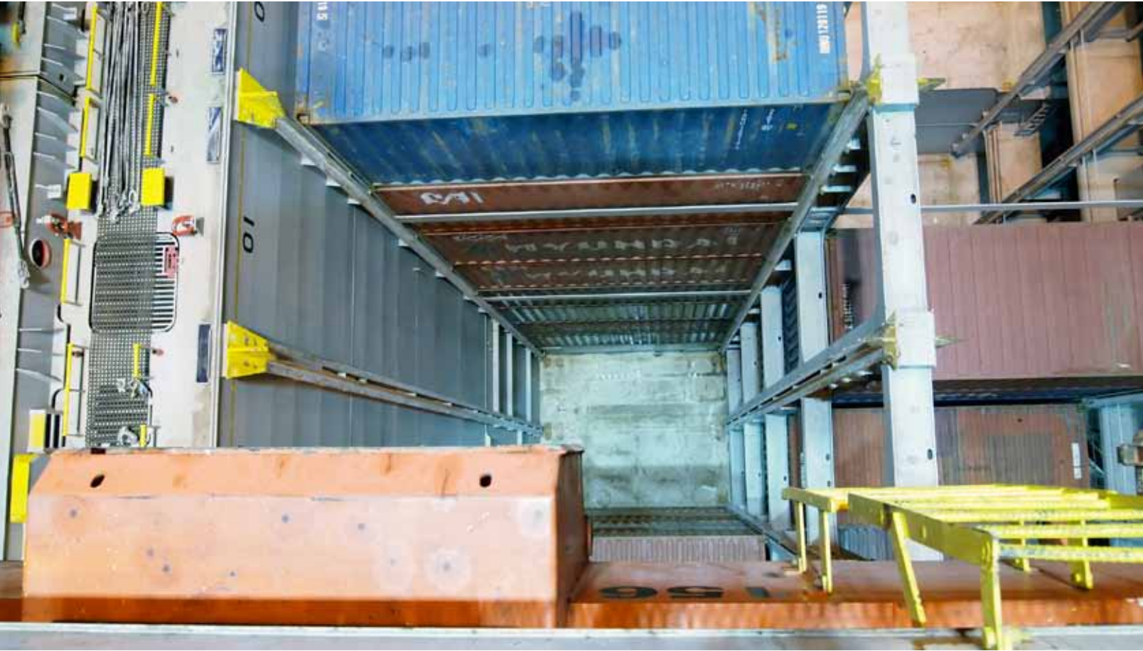
Four 300-watt LED floodlights illuminate all the way to the bottom of a cargo hold, and replace four 1,000-watt HID floodlights.
