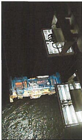
This picture shows four 300W LED floodlights (Phoenix Products - ModCom Hi's) mounted on the trolley of an STS crane illuminating the spreader over the water
