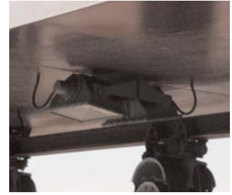
The MRSE Series Heavy-duty floodlight mounted underneath boom of crane
